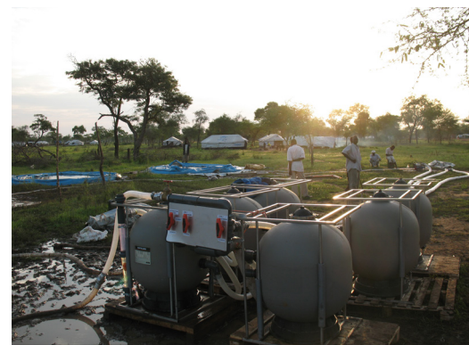
At the Jamam refugee camp, Ali realized that chlorination levels for camp water systems were based on municipal standards.
